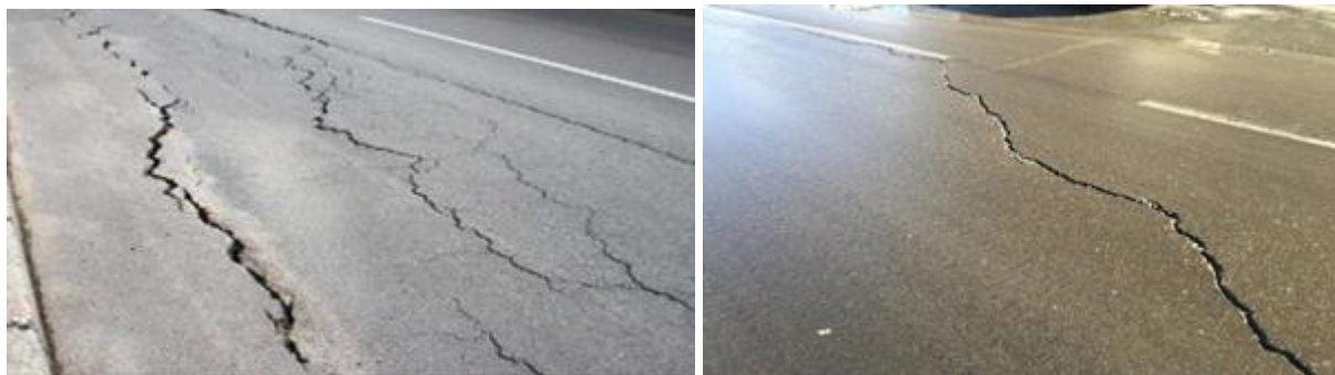
Fig. 2. Disruptions (depth) and cracks caused by deformations in the base layers of the road surface.
