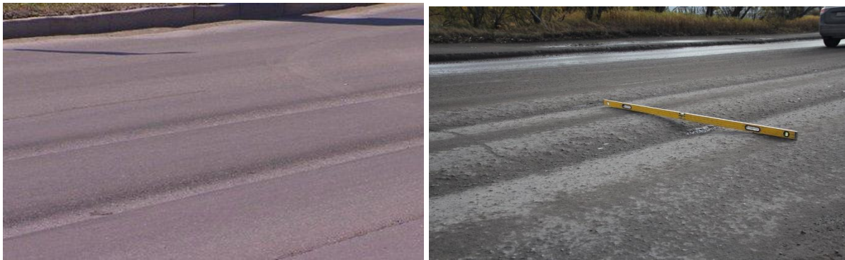
Fig. 1. Deformations of wheel tracks formed on pavements as a result of vehicle movement.
