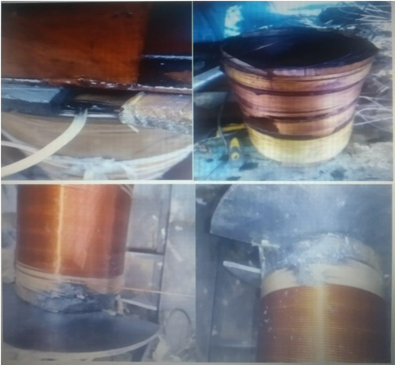
Figure 1. Burned and damaged cases of the transformer core.
