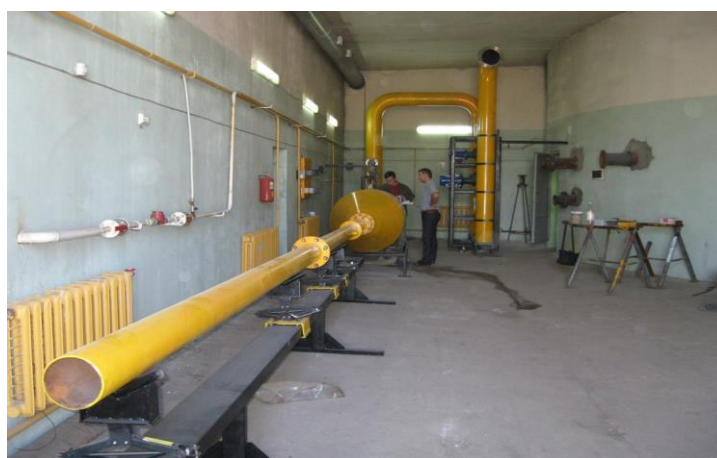
Fig.3. Stand equipped with Roots blowers
